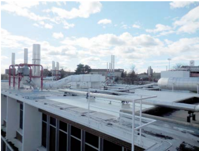
Mechanical systems on the roof show individual fume hood exhausting.
