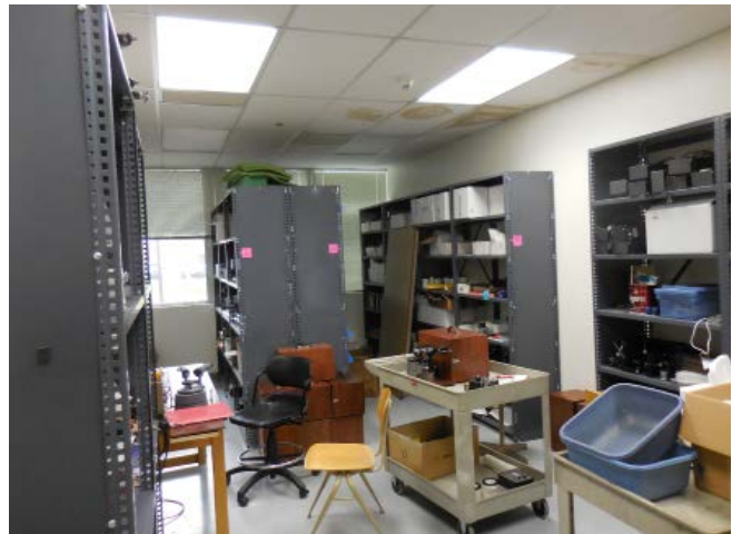
Several spaces in the existing building show evidence of water damage.
